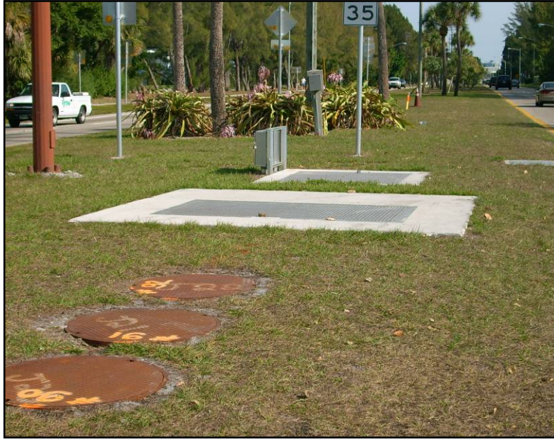
TYPICAL PUMP STATION LAYOUT. 3 MANHOLE RINGS INDICATE BAFFLE BOX, LARGE SQUARE, PUMP WET WELL W/PUMPS AND SMALLER SQUARE IS VALVE VAULT. THIS PUMP STATION ON JOHN RINGLING BLVD JUST EAST OF N WASHINGTON DR.
